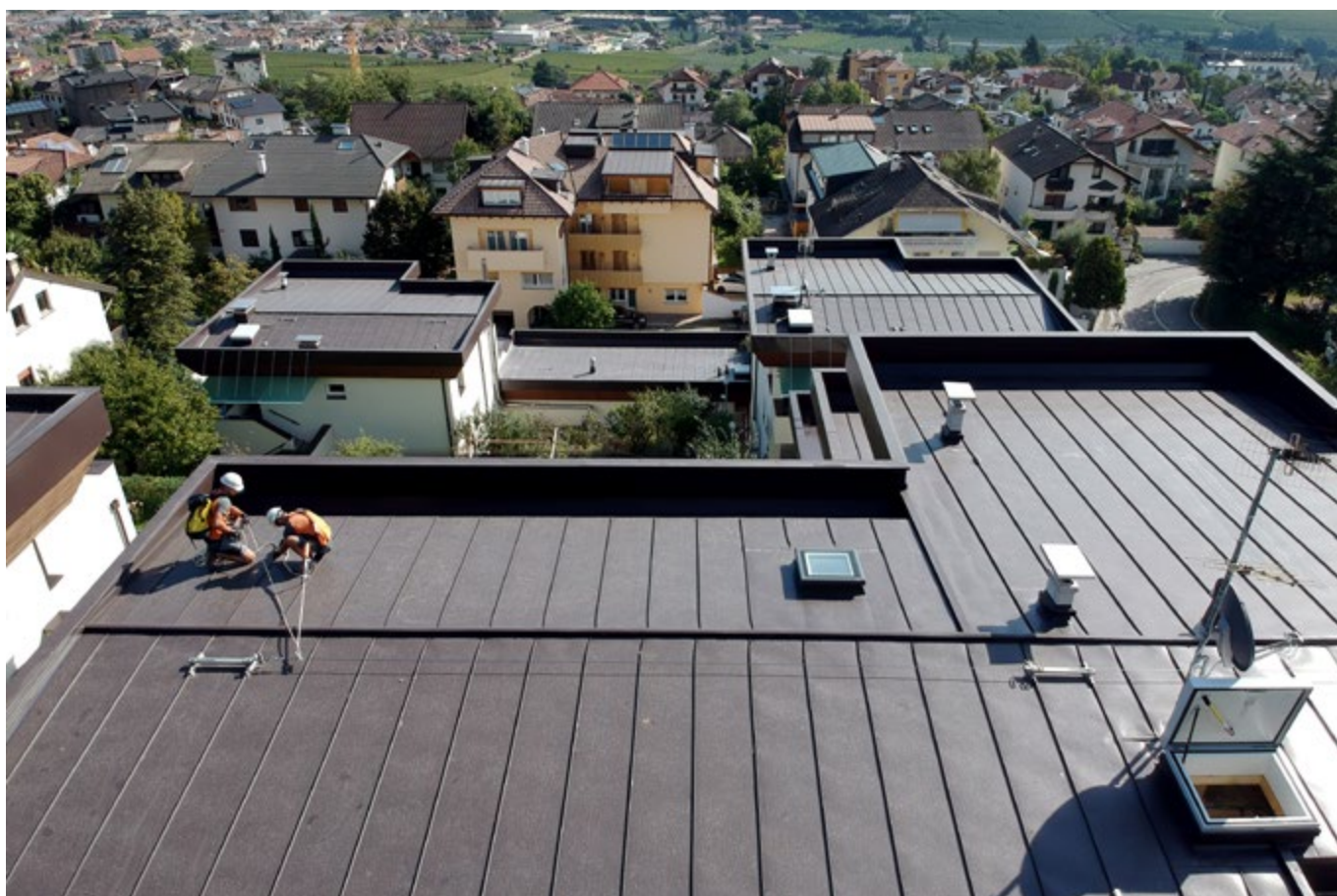
TsSafe for standing seam metal roofs Type 2 on a residential building.
