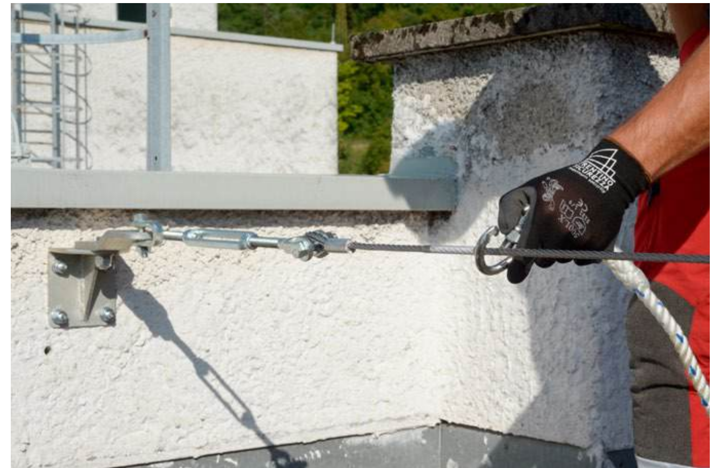
TsSafe with wall plate on a reinforced concrete structure.
