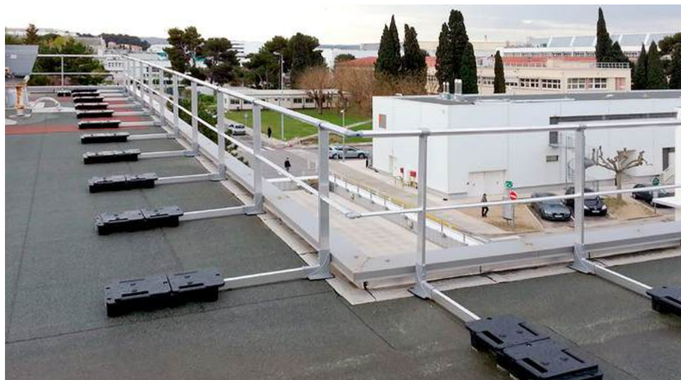
Straight freestanding guardrail.
