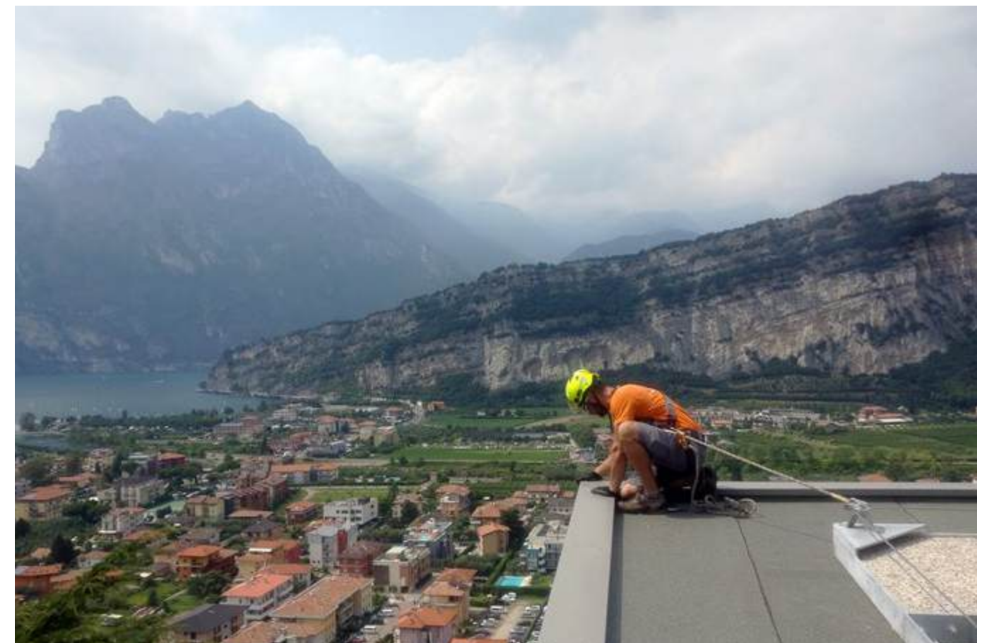
TsSafe with omega plate on a flat industrial roof.
